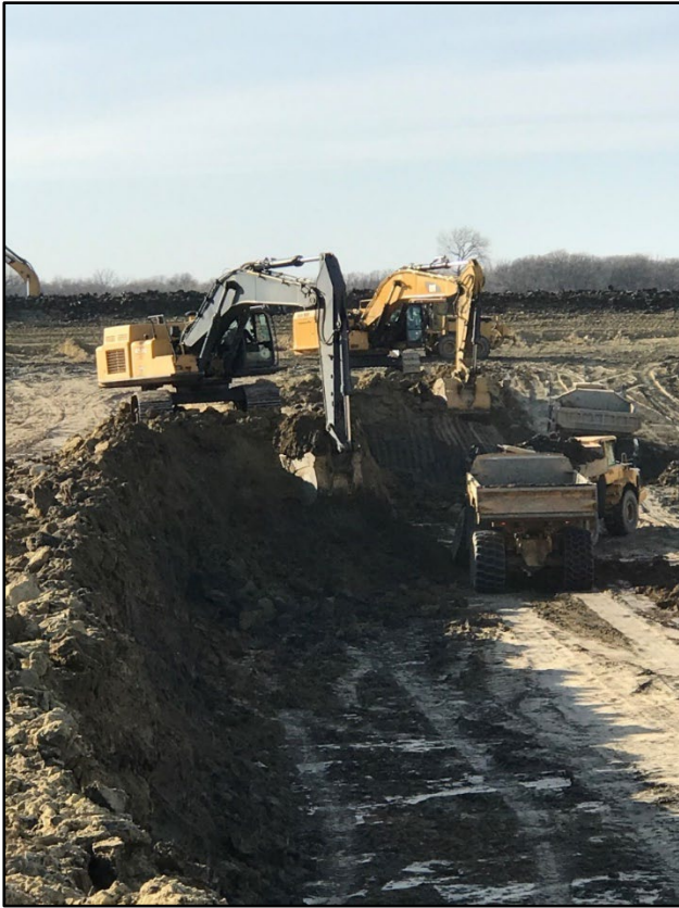
Construction of the Black River Flood Impoundment in the Red Lake WD. Photo courtesy of the RRWMB November 2020.
